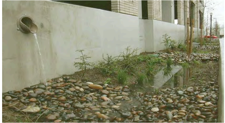
Figure 7: Stormwater Planter with Roof Spout
