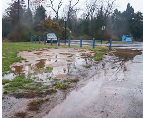
Figure 12: Displaced rainwater runoff
